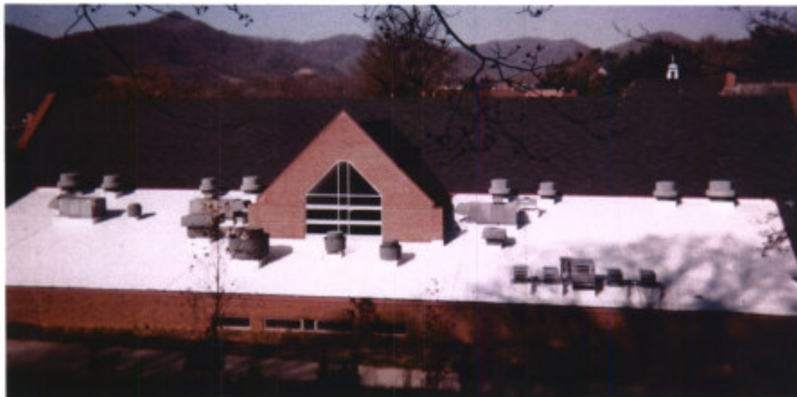
Shown here is the kitchen of Pitman Dining Hall, which used to be extremely hot to work in. Today, the highly reflective white single-ply roof that protects the kitchen also keeps it cooler and more pleasant to work in.
