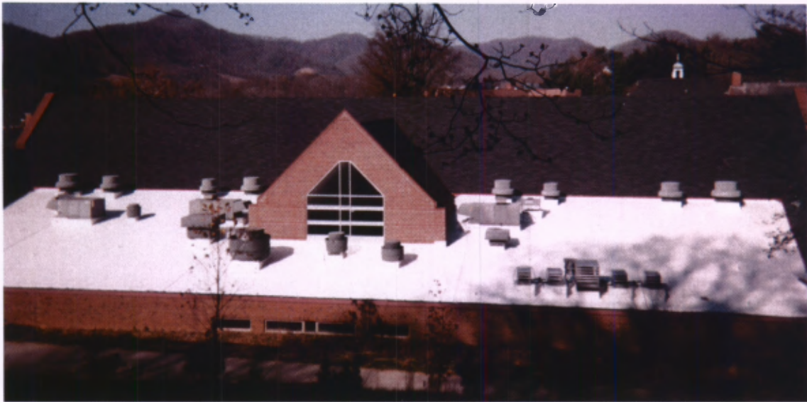
Shown here is the kitchen of Pitman Dining Hall, which used to be extremely hot to work in. Today, the highly reflective white single-ply roof that protects the kitchen also keeps it cooler and more pleasant to work in.
